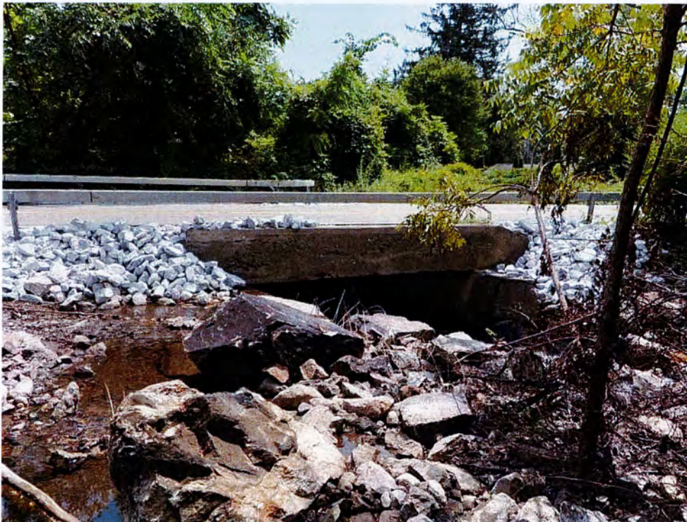
Photo 10. View looking southeast towards the existing culvert, which is slated for replacement.
