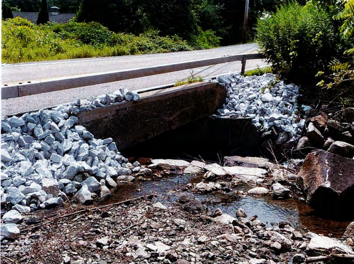
Photo 1. Structure 1, Culvert on Peekskill Hollow Road over Wicopee Brook, looking south. The culvert, constructed in 1925, is heavily deteriorated. The culvert is constructed of metal and concrete, with a concrete and rock retaining wall along either side of the area leading downslope to the Wicopee Brook. The board-formed concrete abutments of this bridge date to 1936. The concrete deck and rails were replaced in 1960. It has previously been determined to be not eligible for listing on the National Register.
