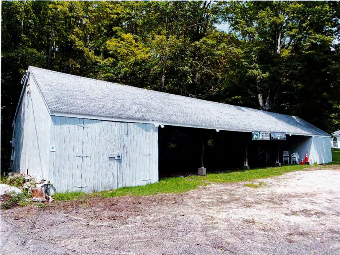
Photo 6. Structure 3a, outbuilding associated with 729 Peekskill Hollow Rd, looking north. Built c.1900, this is a one-story, side-gabled, seven-bay equipment shed. Resting on square posts on concrete blocks, the building is sheathed with flush board siding, and it has an asphalt shingle roof. The two left and the one right bay are enclosed with doors while the center four bays are open. This structure is not eligible for inclusion in the National Register of Historic Places due to a lack of distinguishing features.
